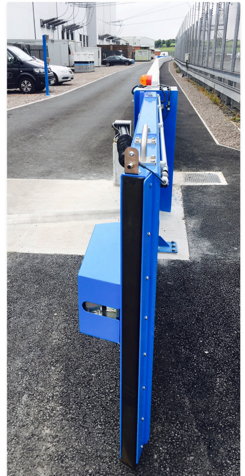
Double swing hydraulic flood gate shown in the open position, with stainless steel cylinder, power pack enclosure and sounder beacon mounted to the gate post.
