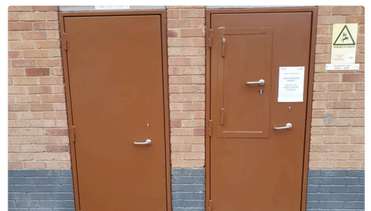
Single-leaf flood doors, one with an integrated access hatch
